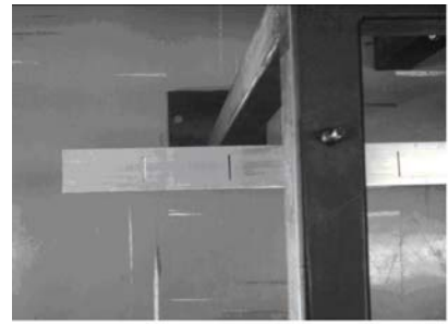
(c) Viga com Dano
