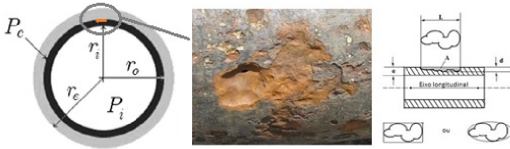
Figure 3: Pipe with metal loss under pressure with a composite reinforcement sleeve.
