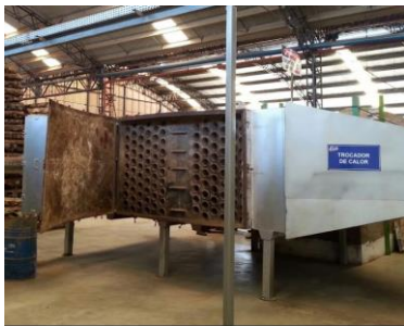
Figura 4. Current heat exchanger at Baldo S.A.
