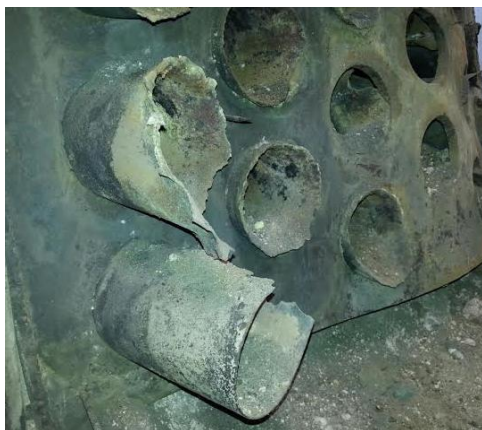
Figura 13. Generated failure by thermal radiation on heat exchanger tubes.
