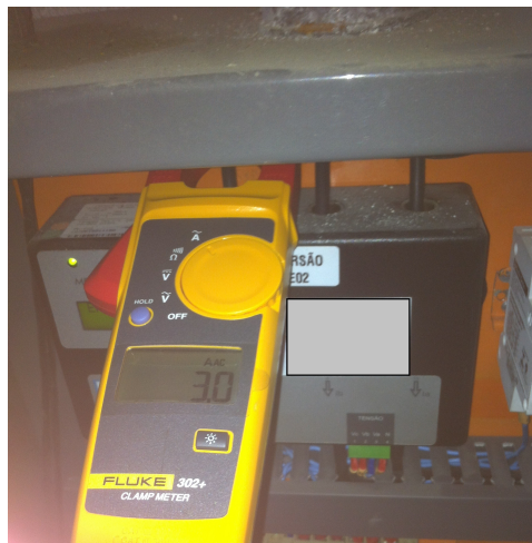
Figure 1. Electrical current measurement using the Clamp meter.
