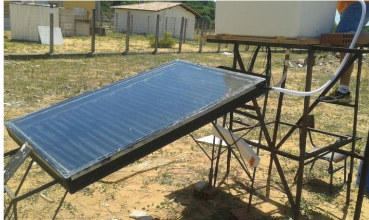
Figure 2. Solar collector in the test.
