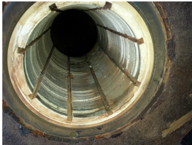
Figure 6. Polymer lining damage
