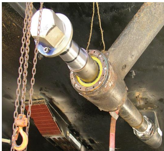
Figure 2. Supports of the propeller shaft
