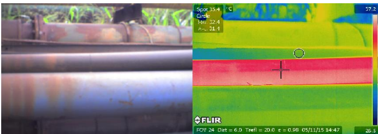
Figure 9. Pipe carrier coal slurry and your corresponding thermal image
