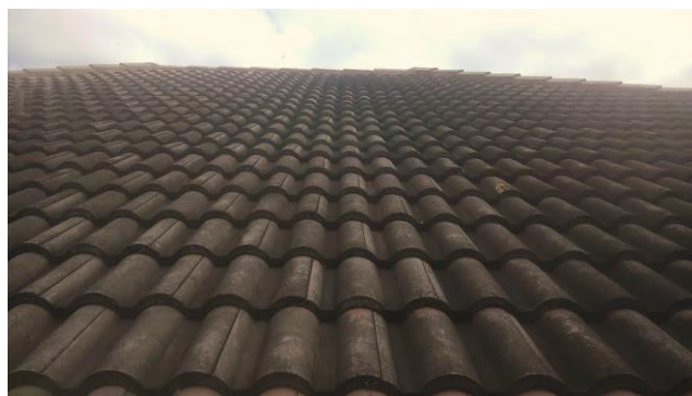
Figure 1. Mould Growth on concrete tiles.
