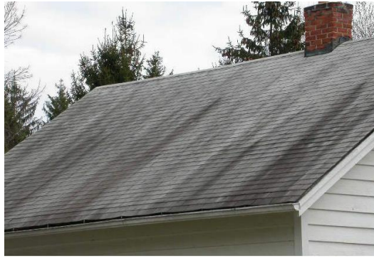
Figure 2. Mould growth on asphalt roofing shingles.
