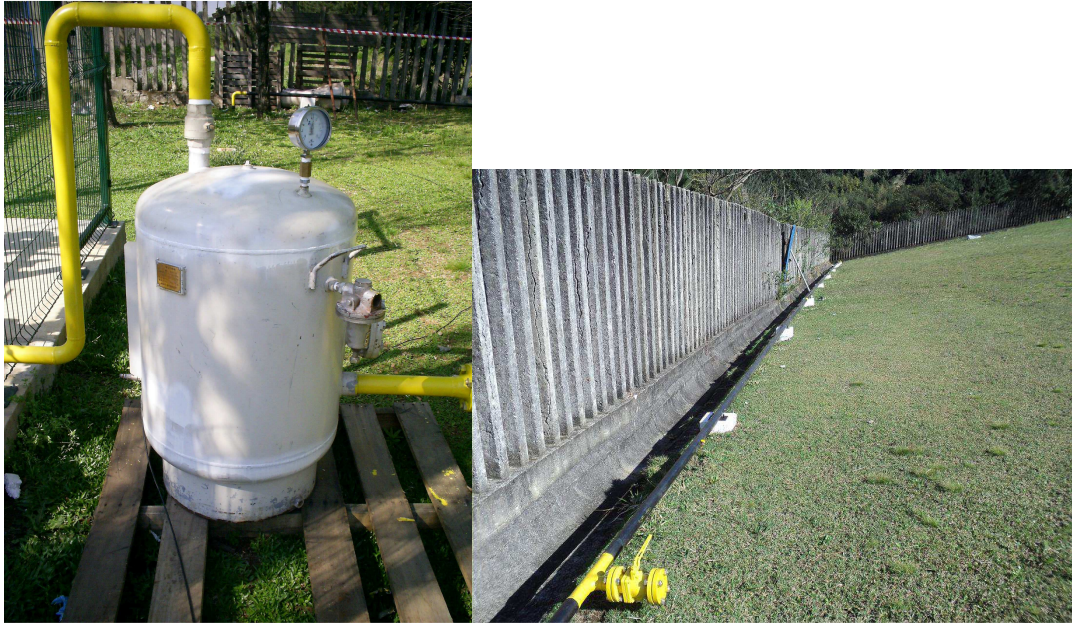
Figure 4. The pressure vessel and main pipeline
