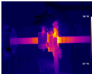
Figure 4. Thermal photo of the coupled bearing
