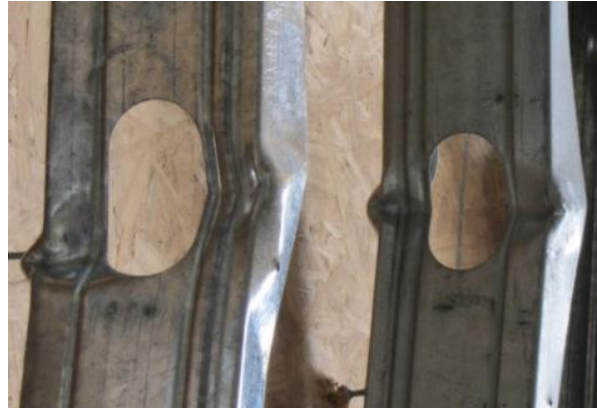
Figure 10. Buckling of the stud in the region of the holes
