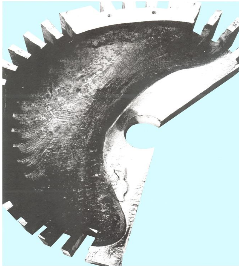
Figure 3. A very deep crack which has developed in a 320 MW generator.
