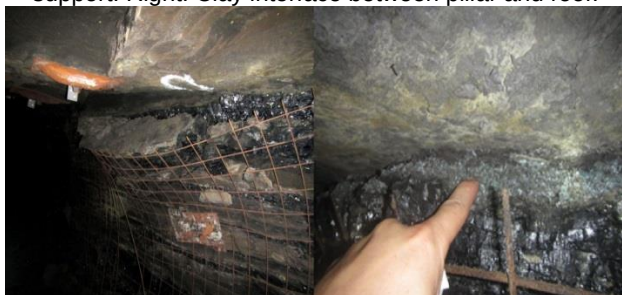
Figure 1 Left: Pillar damages and steel mesh used for support. Right: Clay interface between pillar and roof.
