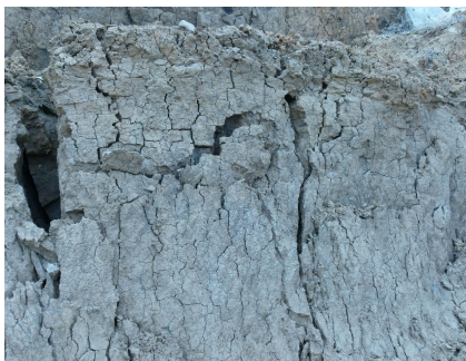
Figure 2. Vertical fissures of surface soil
