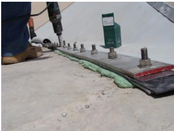
Figure 1. Sar Cheshmeh GFRD, Iran 2008. Perimeter seal of the tie-down type at abutments.
